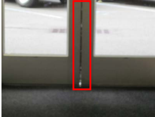
Exterior door in need of weather-stripping
